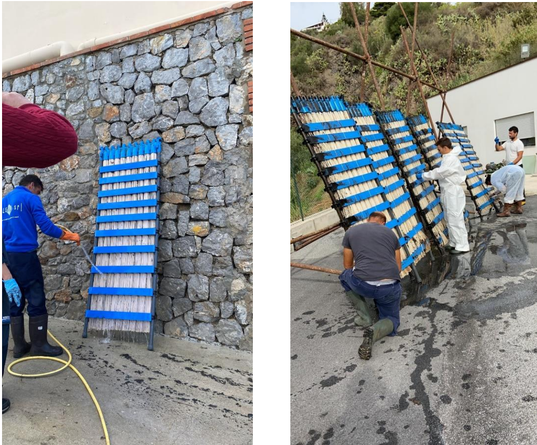
Fig.3 manual cleaning of membrane rows with water hoses
